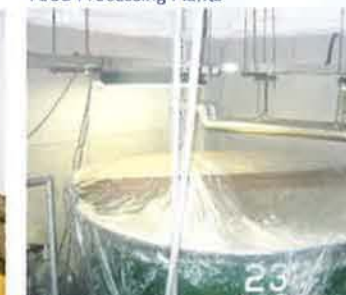
Air purification at a sake brewery
